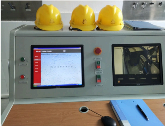
PIC 2. Control device of PR2 testing system
